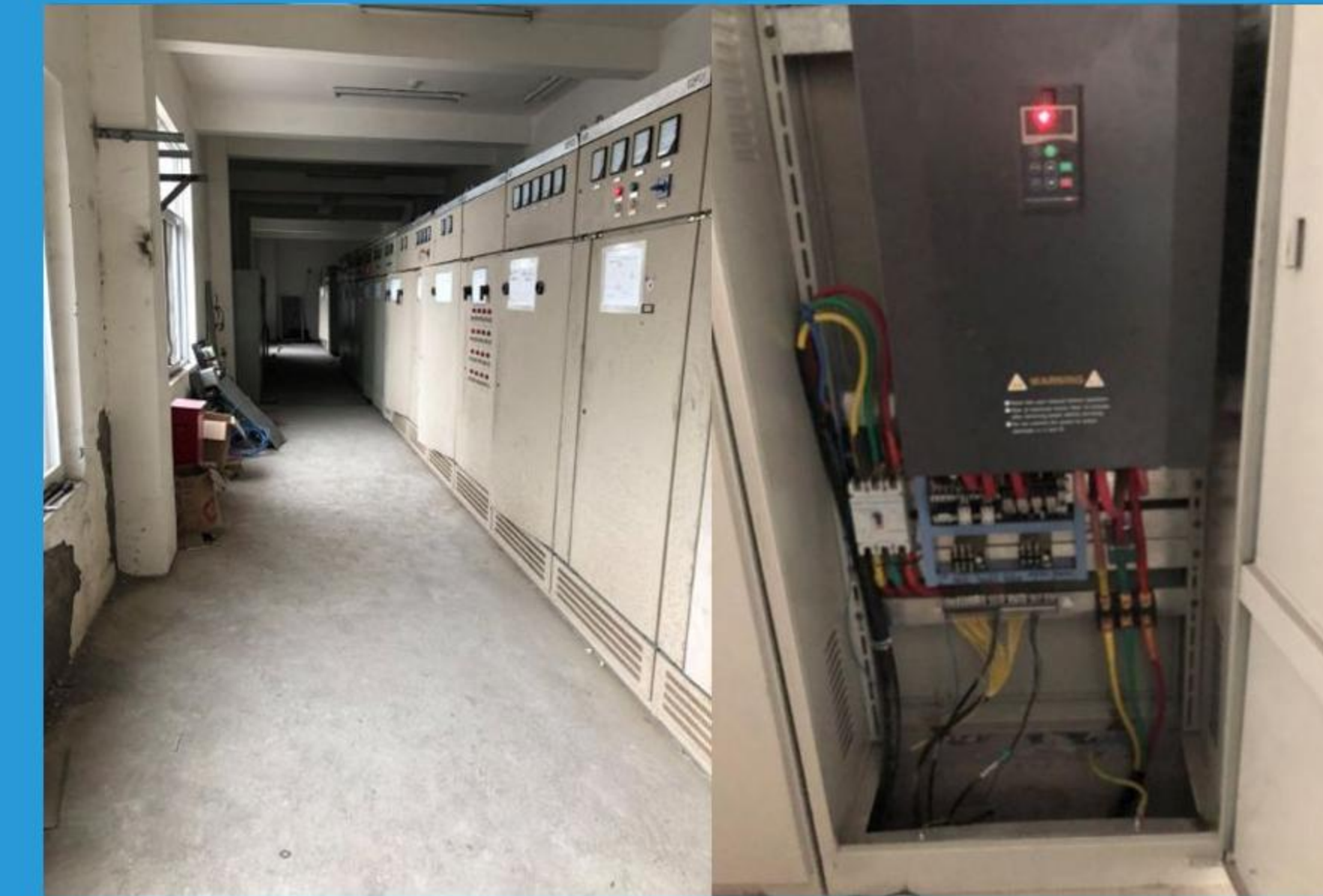
Power distribution management
